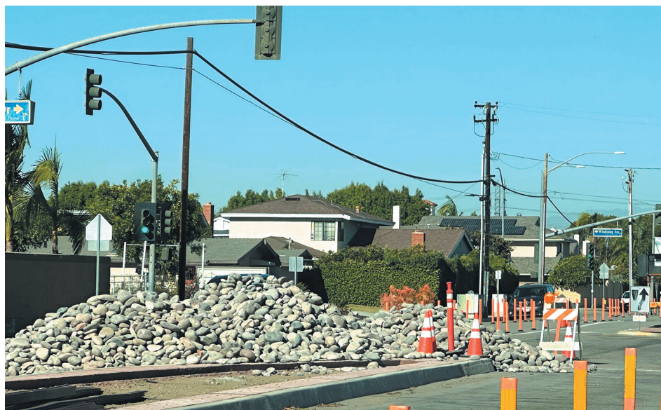
THE PROJECTS are along Walker Street, between Orangethorpe Avenue and Bransford Drive; Moody Street, between Houston Avenue and Crescent Avenue and La Palma Avenue, between Denni Street and Valley View Street.
