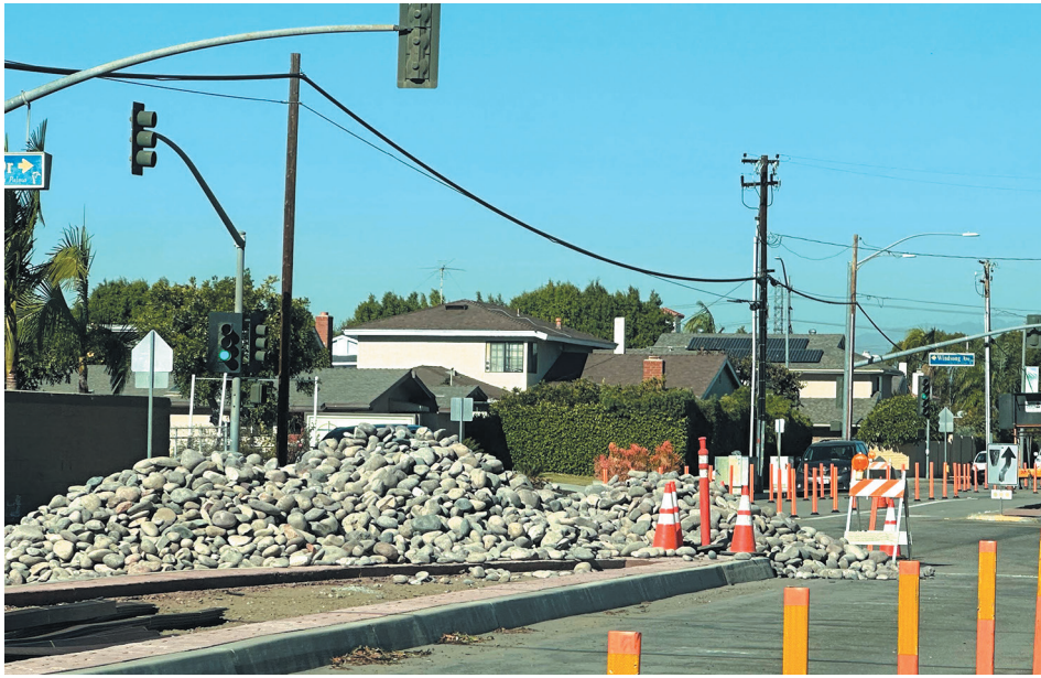
MEDIAN WORK in La Palma. The additional funds will cover the installation of a river rock bed and additional concrete “sleeves” between median islands. Improvement work includes Walker Street, between Orangethorpe Avenue and Bransford Drive and Moody Street, between Houston Avenue and Crescent Avenue.
